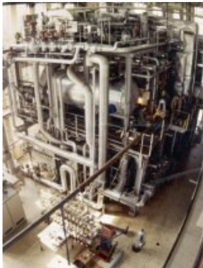
KEMA experimental boiler installation
