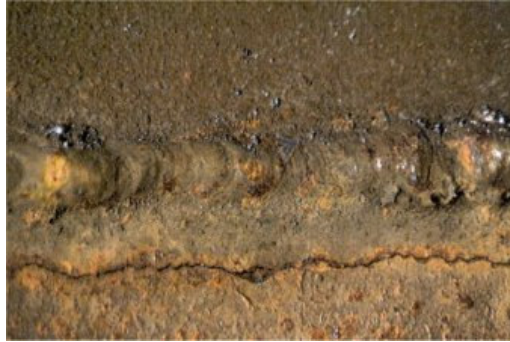
Figure 1. A cracked zone near the weld.
