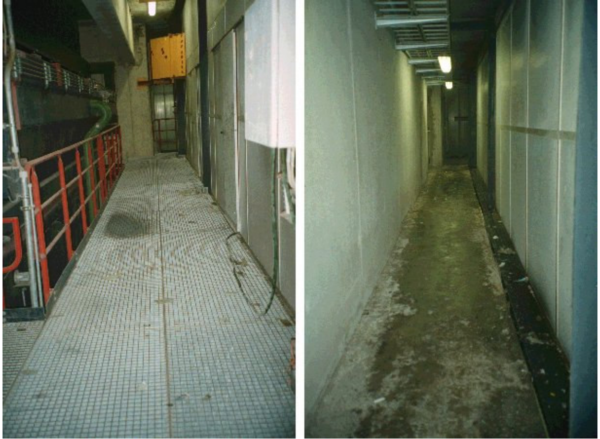
Figure 1 Corroded galvanised gangways
