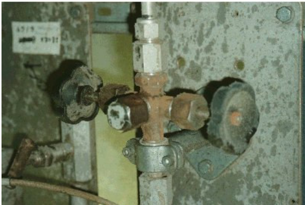
Figure 3 Corroded aluminium isolation plates and steel valves
